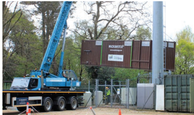
The 40-foot Muckbuster installed at the University of Southampton Science Park receives source separated food waste and some green waste.
